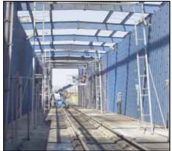
Up to 14 new spinner nozzles on each array in the LMIT locomotive wash building, plus changes to water pressure, contribute to cleaner locomotives.
