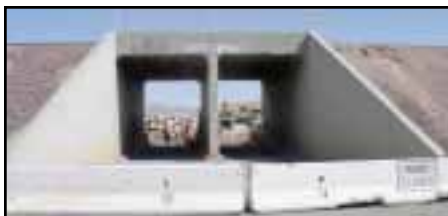
Closed for construction, this bridge at the west end of Barstow Yard undergoes widening for a third main line track.
