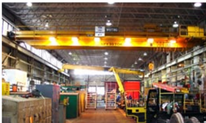
Crane America Services crews operated a forklift Feb. 8 to install a new 10-ton crane on Line 4 and 5.
