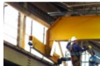
A crew member helps guide the 63-foot crane into place. Extensions were added to the crane’s body to ensure its ability to lift car bodies from locomotives.
