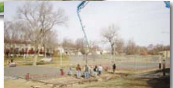
The concrete surface of the new Eagle Park basketball court is poured.
