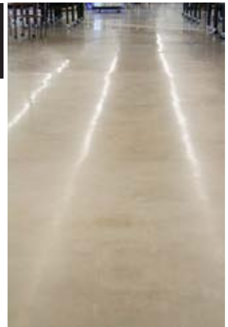
Omaha's newest Hy-Vee at 144th Street and Stony Brook Boulevard was one of many recent Stephens & Smith projects, where shoppers will travel up and down a Stephens & Smith floor to find their grocery bargains.
